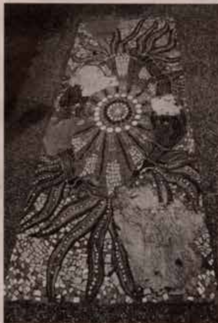
The damaged artwork at Jilli Binna which has now been totally replaced by a cement slab
