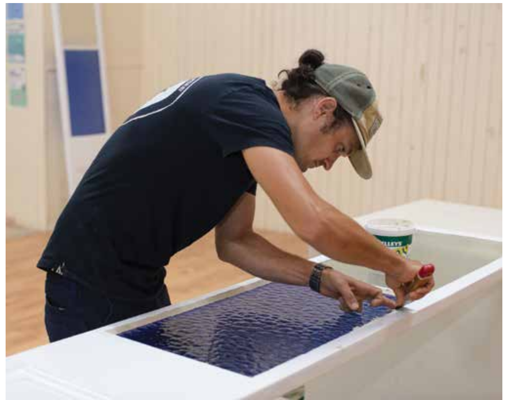
Ongoing Hall renovations include restoring the coloured windows. Clayton Crowe from Nailed IT maintenance, is working on the hall doors with blue stained glass. This blue colour is Pantone PMS280C.
