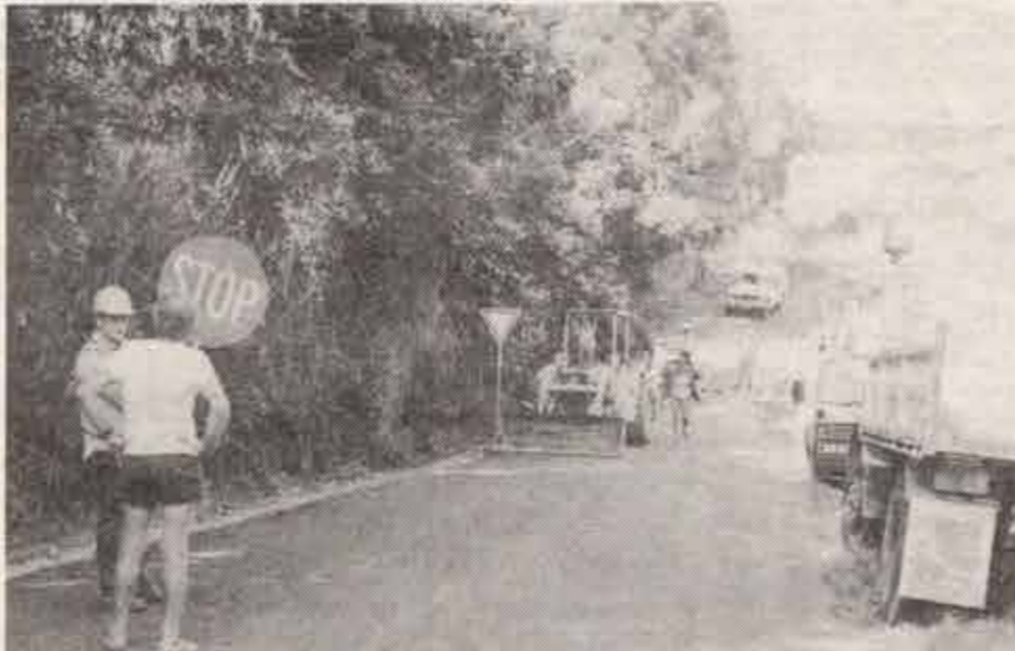
Timely repairs to the Myola bridge, cause inconvenience for some but an opportunity for a chat for others.
