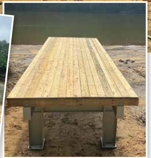
Top: The Barron River esplanade where the Kuranda Riverboat jetty used to be. Left: Kuranda Riverboat owner Warren Clinton rebuilding the jetty. Above: The rebuilt jetty April 2024. Photos: Kuranda Riverboat
